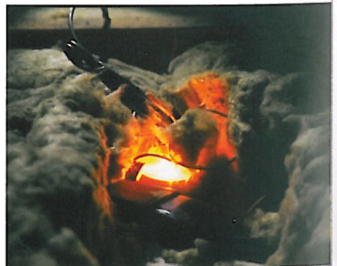
Insulation too close to a downlight.
